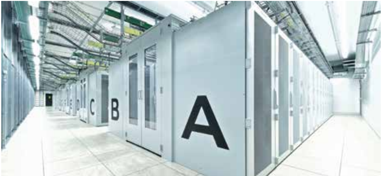
Audi's new data centre at the Ingolstadt plant provides 2,000 square metres of space for 6,000 highly efficient servers. The TÜV Rheinland technical inspectorate has issued the data centre with a "premium" certificate – its highest energy efficiency rating.
