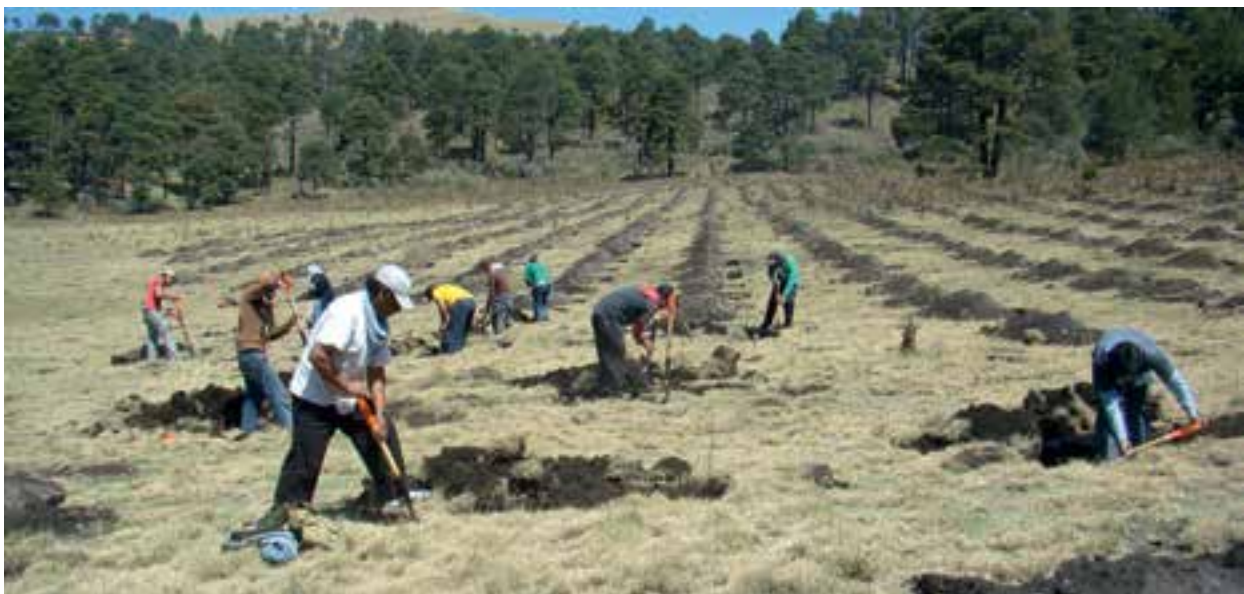
Tree-planting under way on mountainsides in the Iztaccihuatl-Popocatepetl National Park. In the course of this reforestation project, 420,000 trees have been planted, 47,000 soakaways have been dug and 350 sizeable dams have been built to date. These measures are contributing around 2.6 million m 3 to groundwater replenishment annually.
